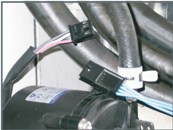
Image 13-24 Electrical connection pump
